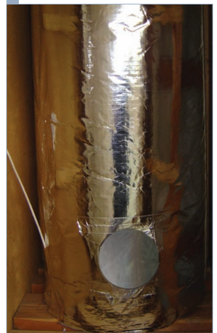
9 Control panel access left exposed
